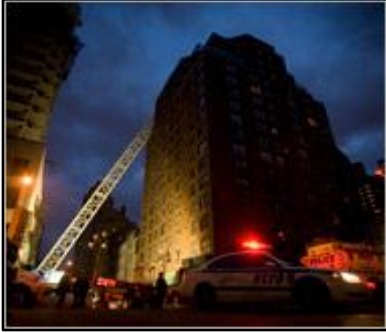
Part of a construction crane remained leaning across the street Saturday night after it toppled, crushing one building and damaging others on the East Side of Manhattan.
