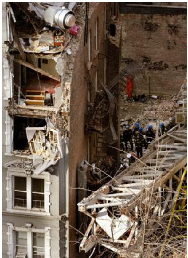
Rescue workers search through wreckage of a crane collapse on 50th Street near Second Avenue in 2008.
